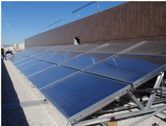
Picture of the collector field
