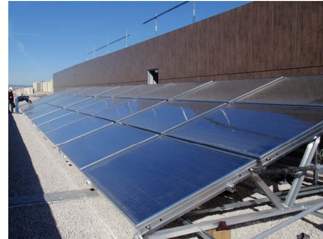
Picture of the collector field
