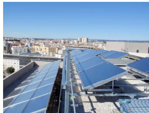
Solar collector fields in drainback mode
