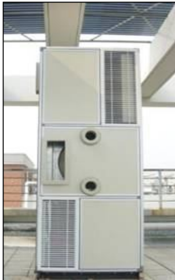
Rotary desiccant cooling(2007)
