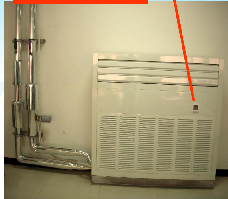
Embedded fan coils in restaurants
