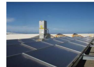
Solar cooling installation for a Tertiary building in Tropical climate (Source: TECSOL)
