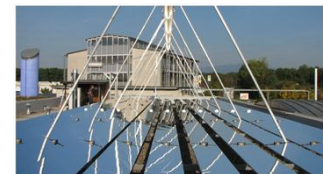
Fresnel collector field adapted for solar cooling (Source: Industrial Solar GmbH)
