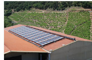
Solar cooling installation for a wine cellar in the south of France (Source: TECSOL)
