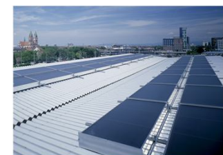
Solar cooling installation using DEC technology and air collectors in central Europe (Source: Fraunhofer ISE)
