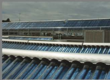
Echuca Regional Health solar cooling system with Greenland tubes
