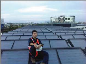
UWC-SEA building solar cooling project in Singapore by SOLID
