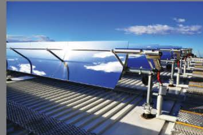
Charlestown Square Solar Cooling
