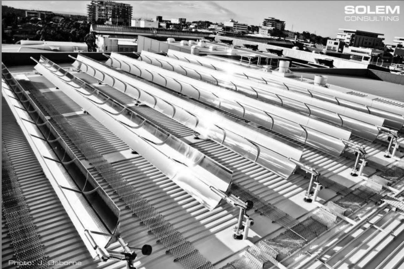
NEP Solar - Charlestown Square Solar Cooling Project
