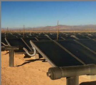
39,000 m2 flat plate field in Chile CODELCO copper mine
