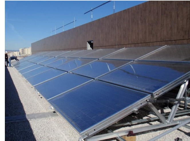
Picture of the collector field
