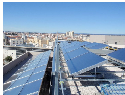
Solar collector fields in drainback mode
